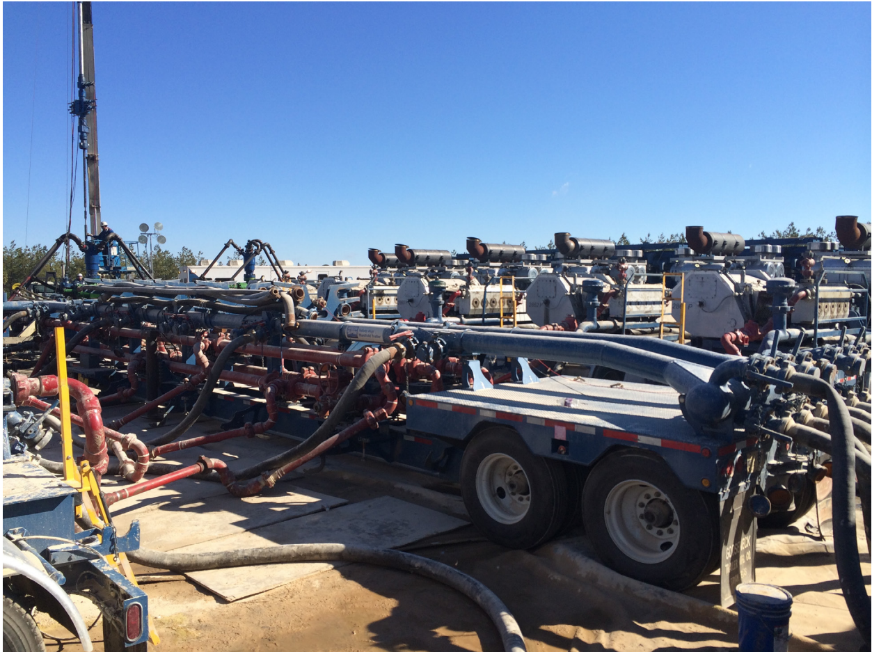
Figure 5-8. Hoses and lines at a site in Arkansas.
