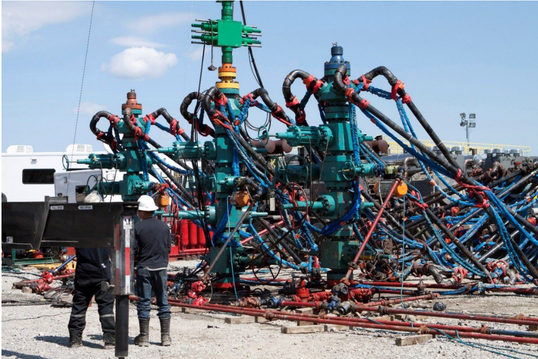
Figure 3-12. Three wellheads on a multi-well pad connected to the piping used for hydraulic fracturing injection.
