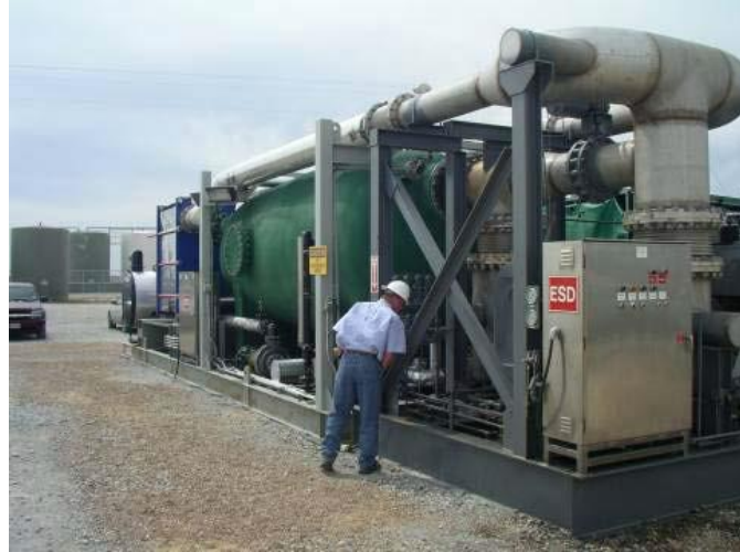
Figure F-4. Picture of a mechanical vapor recompression unit near Decatur, Texas.
