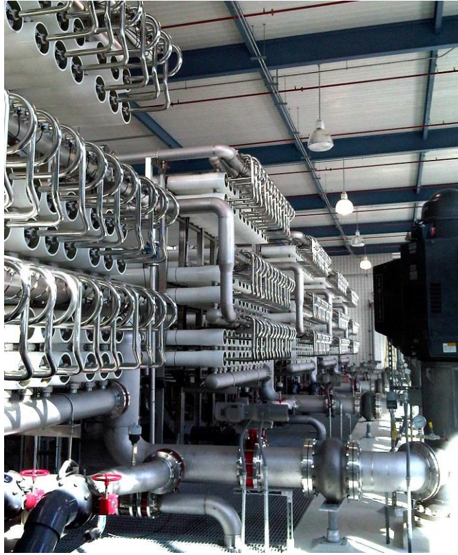
Figure F-2. Photograph of reverse osmosis system.
